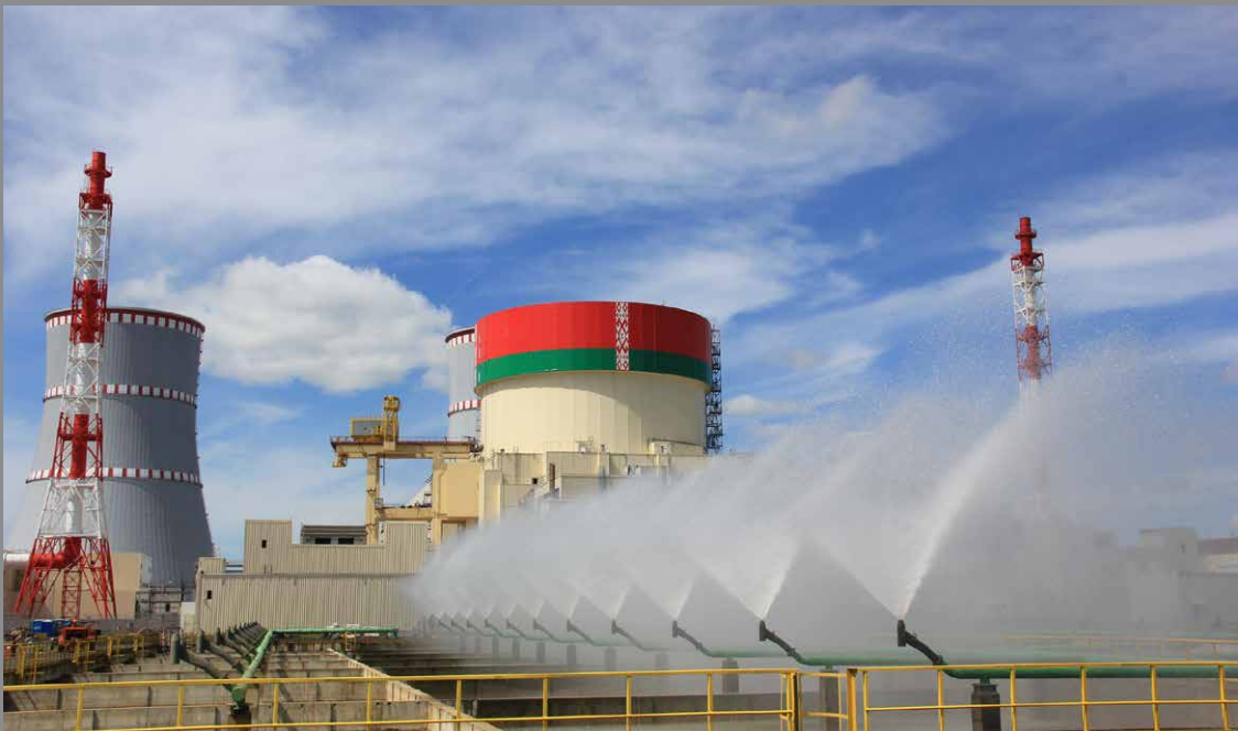
Belarusian NPP. Spray pools consist of four 18,000 m 3 ferroconcrete tanks. All the tanks are equipped with systems of pressure pipelines apportioning the chilled water among the spraying nozzles.
