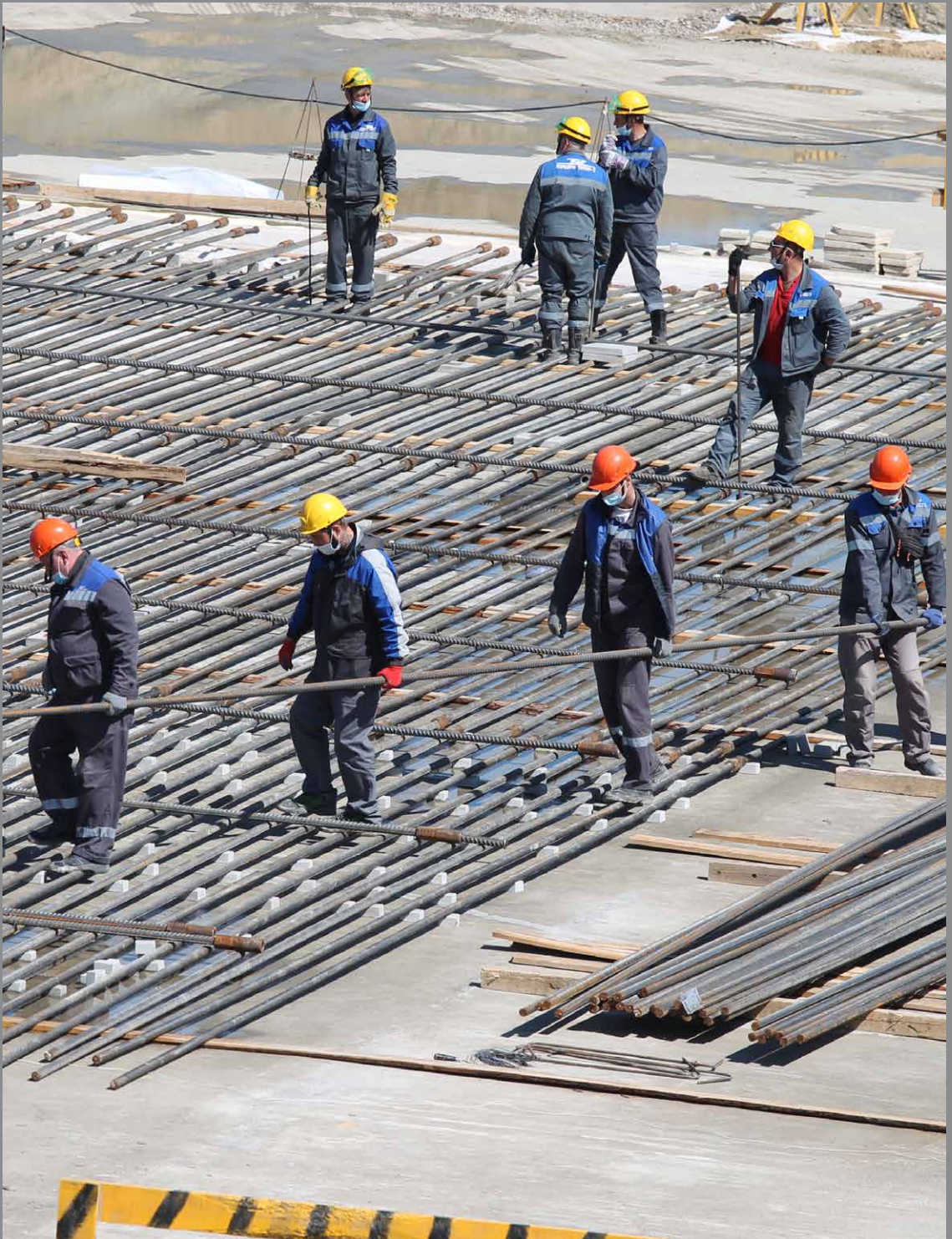
The pouring the first concrete of the BREST-OD-300 reactor of the Proryv Project
