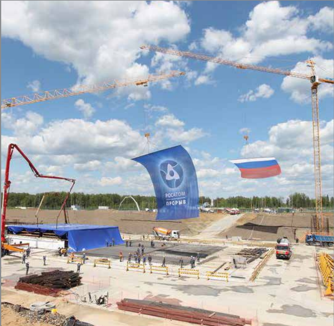
The ceremony of pouring the first concrete of the BREST-OD-300 reactor of the Proryv Project
